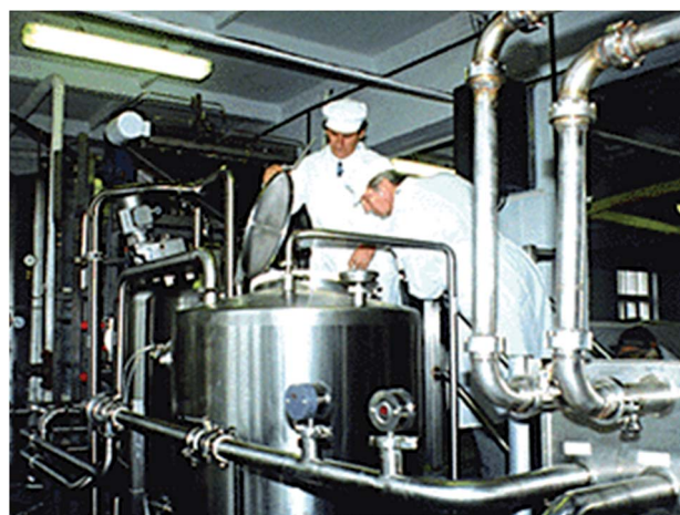
Fig. 5 The MAG*SEP SM milk decontamination system at Ovruch, Ukraine 1997. 1
