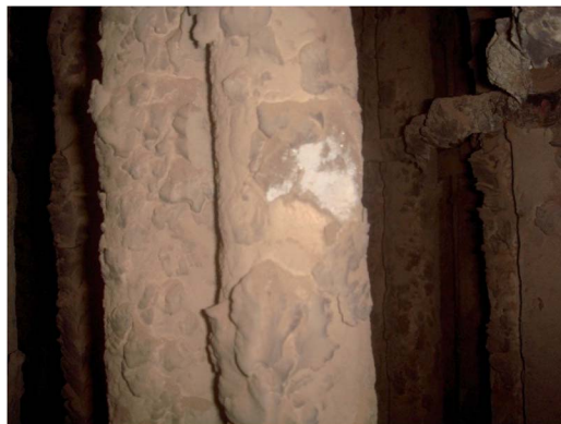
Fig. 2 Deposits on high temperature superheater.
