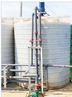
Fig. 6 Chemical solution tank.
