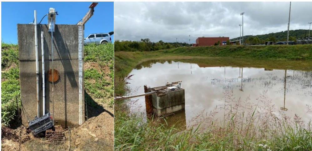
148 Fig. 2. Dry extended detention basin outlet riser (left) outfitted with controllable valve, 149 water depth sensor, and turbidity sensor and (right) the basin following a rainfall event. 150 151
