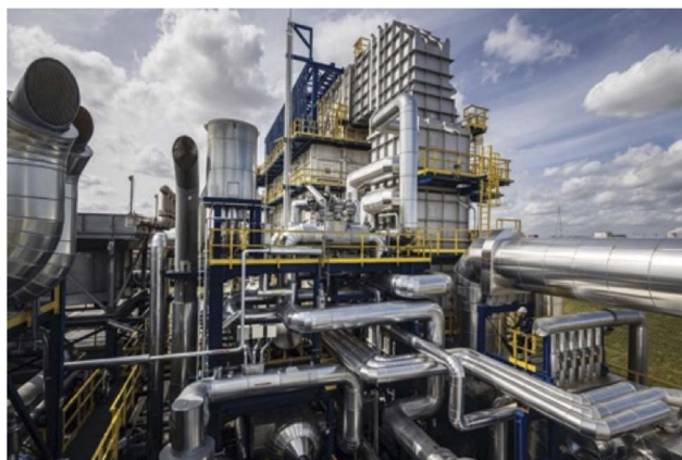
Fig. 14 One of the recent SMR-based H 2 production facilities (Air Liquide's SMR-X process) in Antwerp, Belgium, produces 99.99% pure H 2 at a rate of 56000 N m 3 per hour. The plant went into operation in April 2021. This shows the complexity of the plant and the stainless steel structures required in the form of pipes which carry hot gases.
